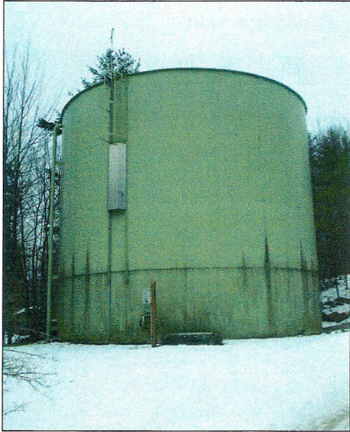
Figure 2. Maple Ridge Water Storage Tank
